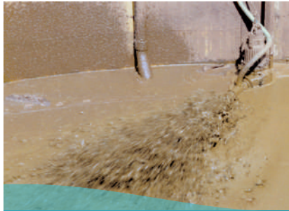
Liquid manure pumps
