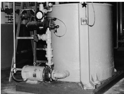
Reverse osmosis, Ósmosis invertida
